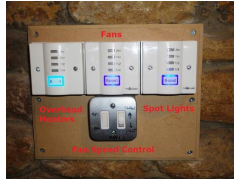
LIGHTS, OVERHEAD HEATERS/FANS located in the kitchen lobby
